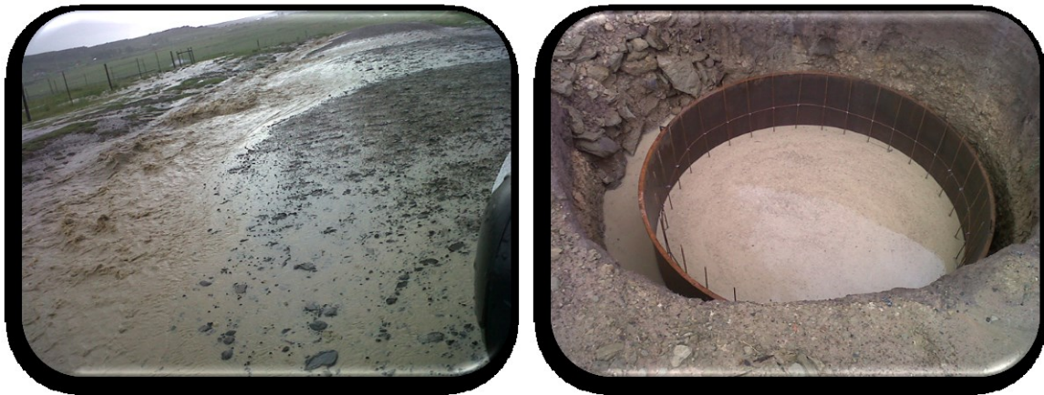
Figure 5-10: Weather conditions can impact negatively upon site access (Left). Figure 5-11: Bio-digester installation delayed due to excessive rain (Right).
