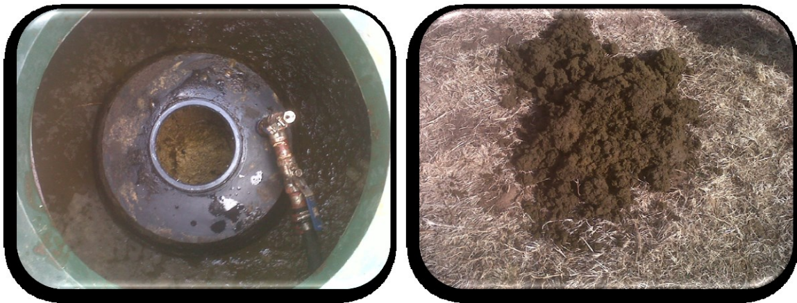
Figure 5-6: Evidence of fibrous deposit within gas chamber (Left). Figure 5-7: Closer inspection of fibrous material (Right).
