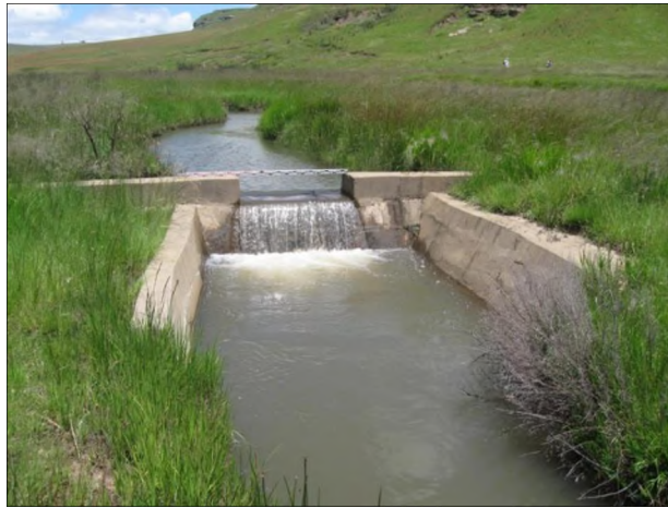
Plate 3.8. View of water back-flooding to the base of an intervention in Killarney wetland
