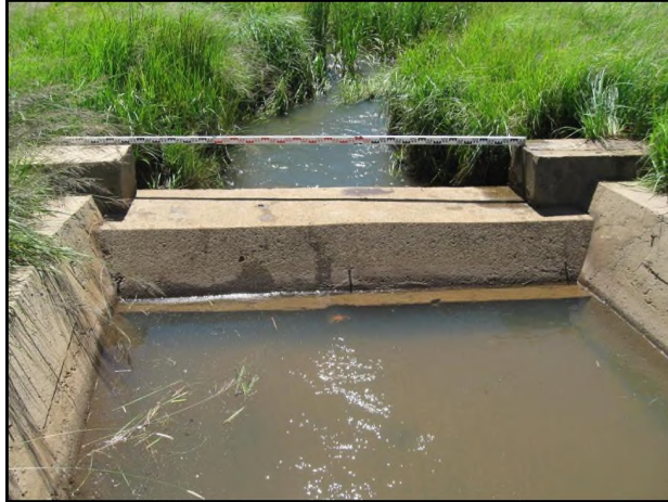
Plate 3.6. View from downstream of an intervention in the Killarney wetland with no water flowing over the spillway as a result of tunnelling that has occurred allowing base flows to pass under the structure.
