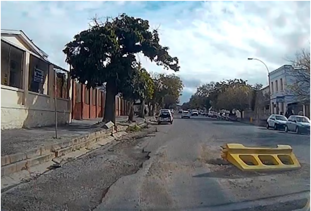
Figure 21: Image of New Street in the Town Area showing road degradation on the left, and a deep pothole with a fallen barricade near the middle of the road. Image taken on 19 September 2018.
