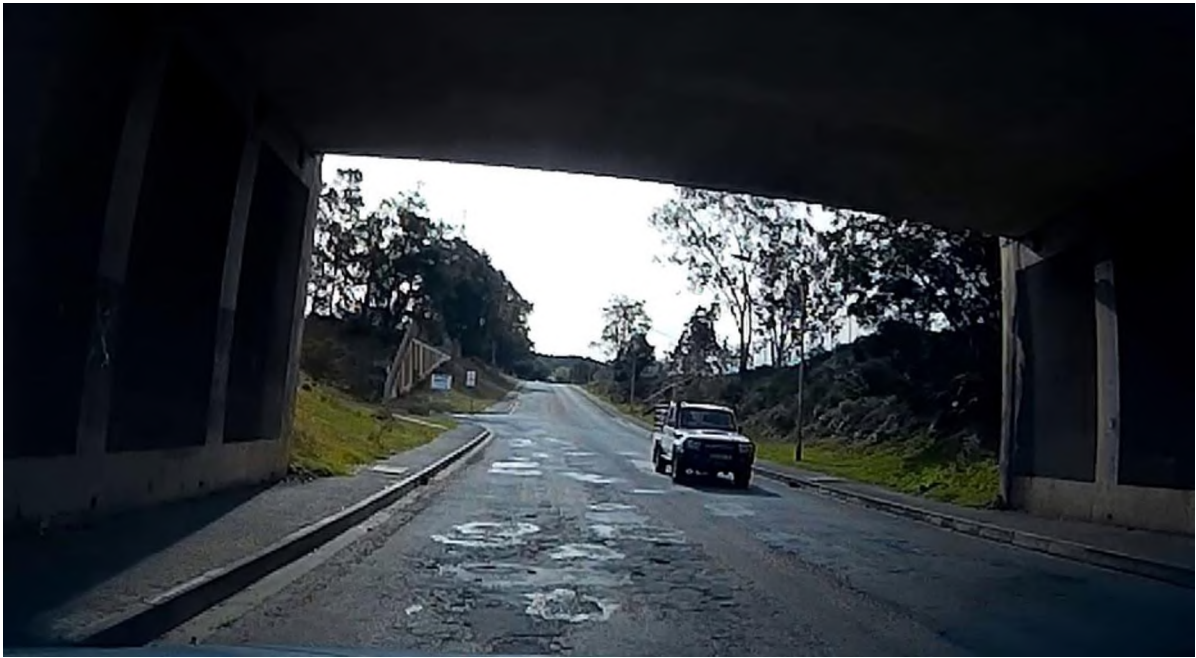
Figure 22: The potholes on upper Milner Street have been filled in several times which has created an uneven road surface. Image taken 17 September 2018.
