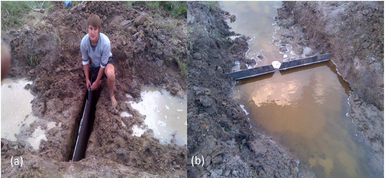
Figure 7: Installation of the V notch weir at the wetland outflow, with the steel sheet v-notch weir in position before opening the channel (a) and after opening the channel (b).
