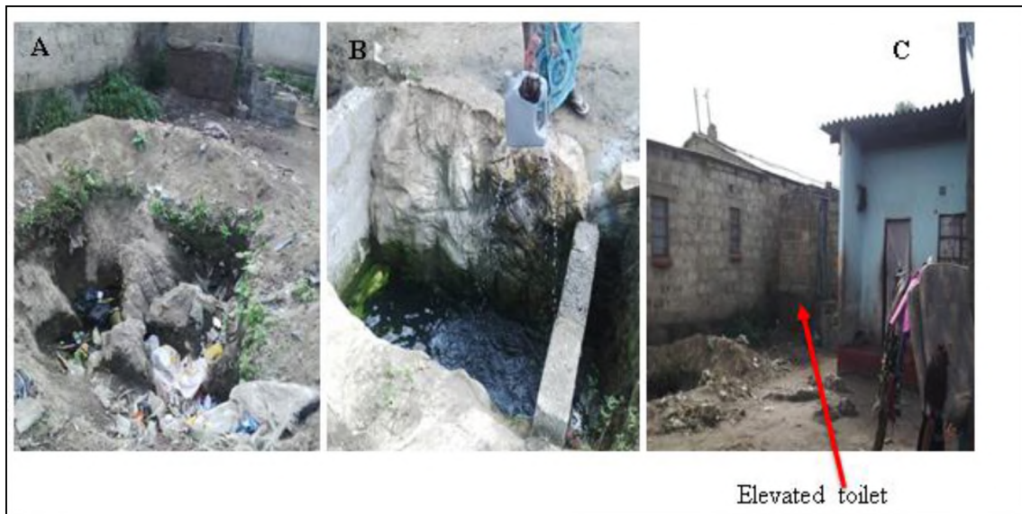
Figure 3.12: (A and B) Pit latrines (just dug out, not elevated) and (C) an elevated pit latrine in Kanyama
