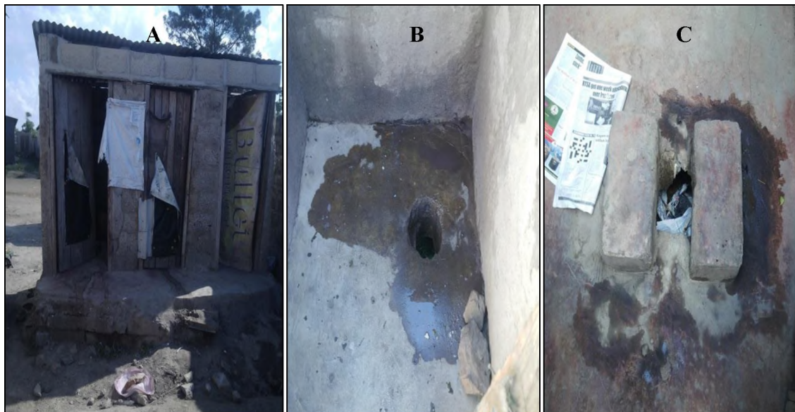
Figure 3.16: (A and B) improperly used toilets and (C).almost filled pit latrine
