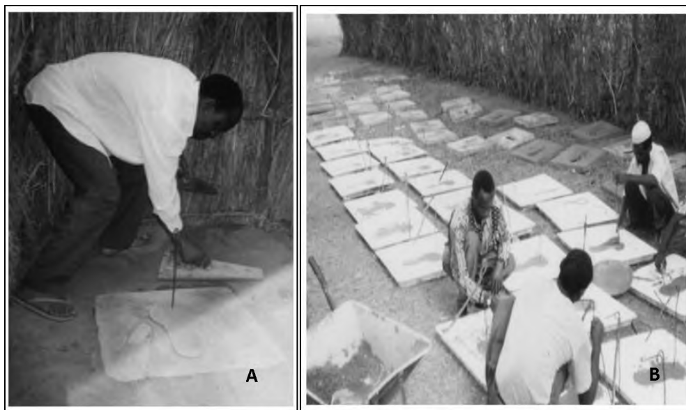
Figure 1.4: (A) A traditional pit latrine fitted with a SanPlat slab and (B) artisans making the slabs (source: Shayo & Chaggu 2004)
