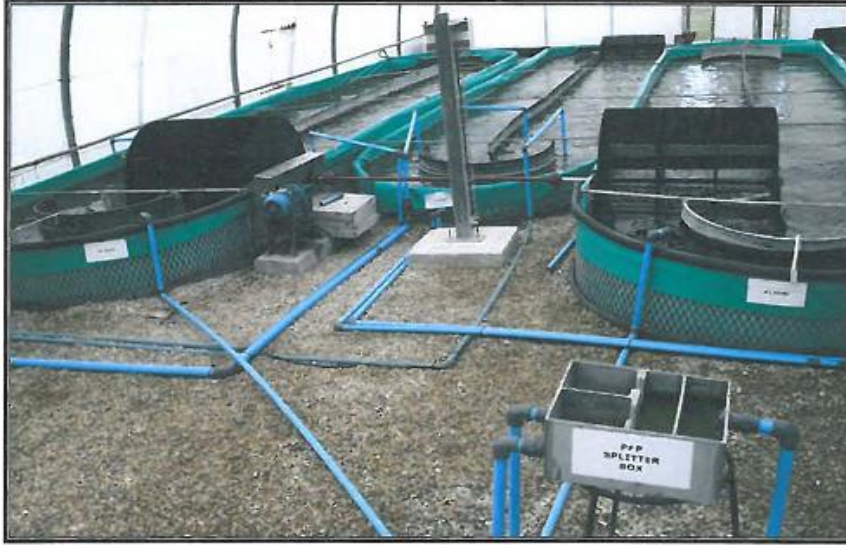
Figure 3: The splitter box directing brewery effluent from the primary facultative pond to the high rate algae ponds (Cilliers, 2012).
