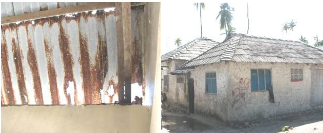
Plate 3.1: On the left, fish market iron-roof corroded by on-shore salt-laden winds. On the right a house roofed using locally-made cement tiles to cope with salt-laden winds in Matemwe, Unguja.
