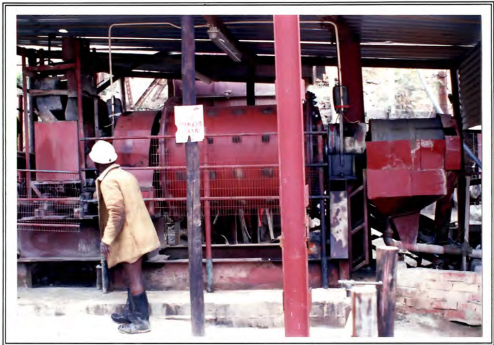
Figure 7.1 Photograph showing a portion of the beneficiation plant at the Dumisa Au mine. The ore is passed through a jaw crusher into a ball mill (center).
