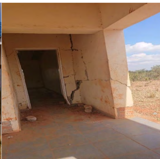
Picture 5.3: VCT Building Damage
