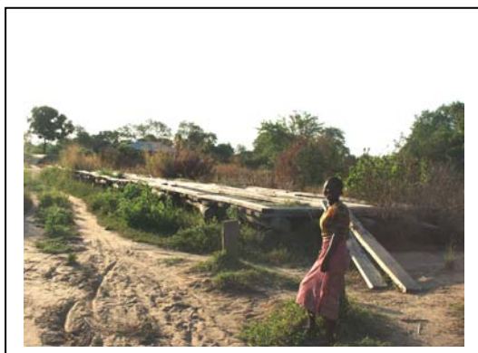
Photograph 1. Bridge left incomplete and rotting
