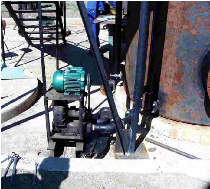
Figure 6.7 The air pump located at the base of the reactor vessel.
