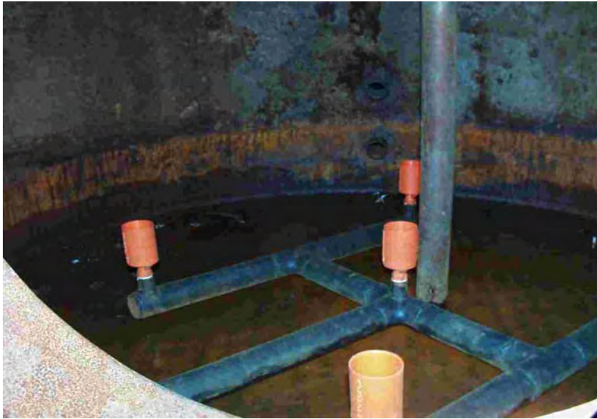
Figure 6.5 The air eductors in the bottom of the reactor vessel.
