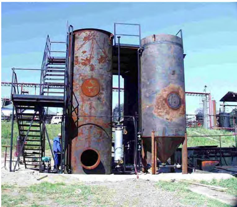
Figure 6.2 The plant upon completion before commissioning.
