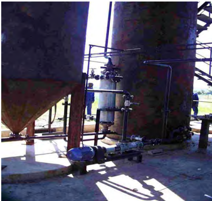
Figure 6.6 Heat exchanger unit located in the recirculation line and feed pump between clarifying tank (on the left) and reactor vessel.
