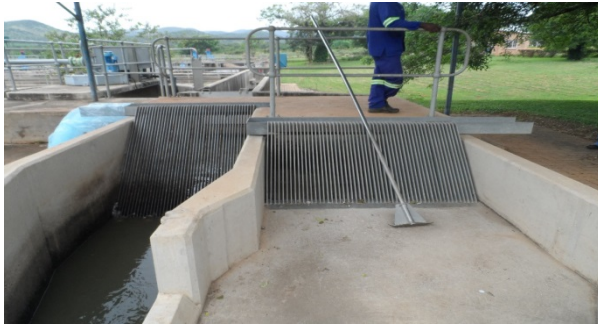
a. Inlet free of debris and screenings properly disposed of
