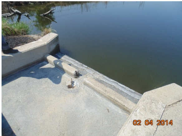
a. Final pond into chlorination channel with no outflow (HTH tablets)
