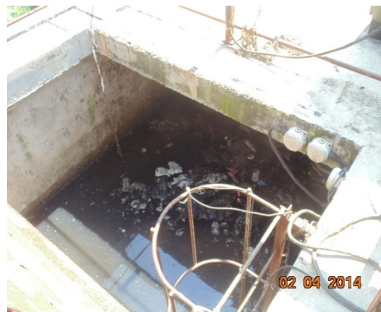
d. Sump full of sewage with no pump
