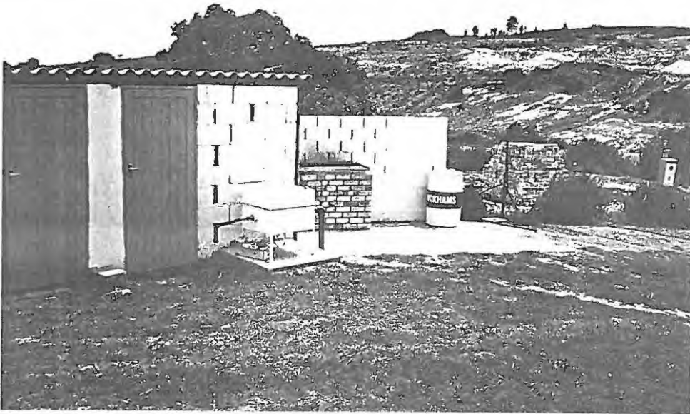
Photograph 2. The Pumphouse with the Condensate Trap in the Foreground.
