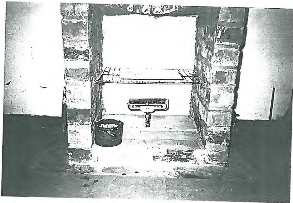
Photograph 6. The Office Heater.
