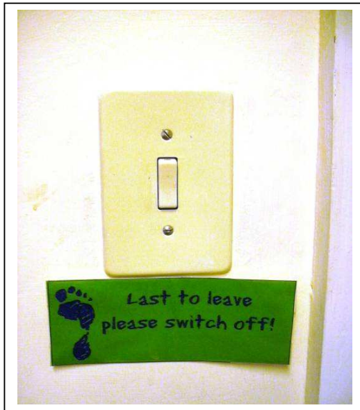
Figure 4.18 A note stuck by a switch in the Faculty of Education
