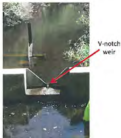
Figure 4.20. V-notch weir in the lower reaches of the Duiwe River which is the freshwater source to Island Lake, Wilderness Lakes system, Western Cape.
