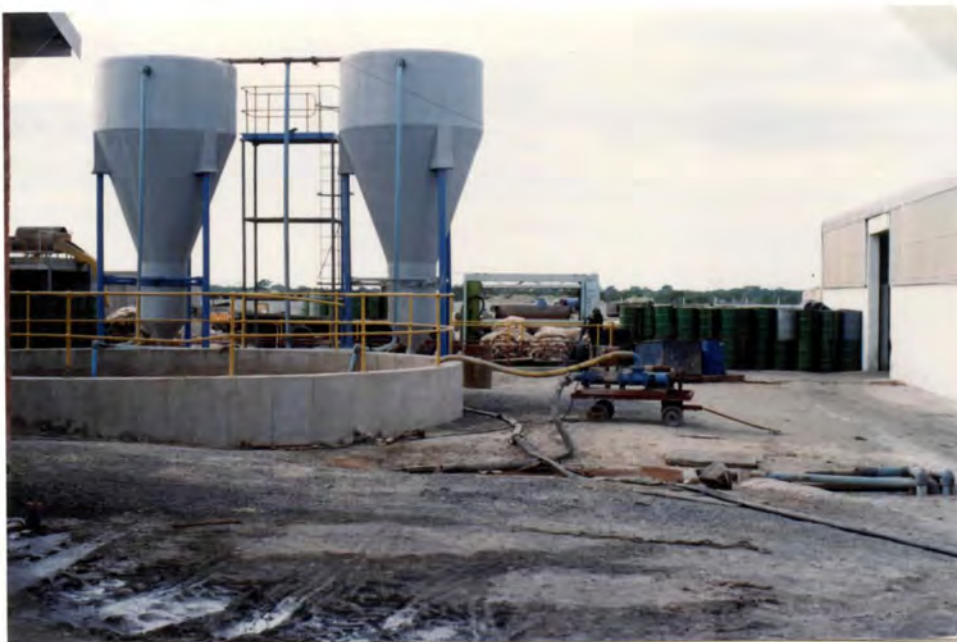
Plate 2.2. The sulphide oxidation tank (circular tank) from which the effluent was removed for use in hydrolysis. Also visible are the two settling cones in which the alkaline effluents were initially settled following discharge from the tannery.
