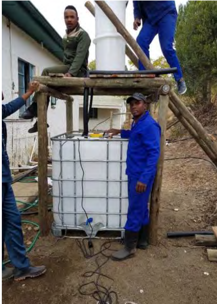
Picture 4.1: Crop Production students and Mr Matambo constructing a grey water harvesting demonstration system. Photo credit - Matambo
