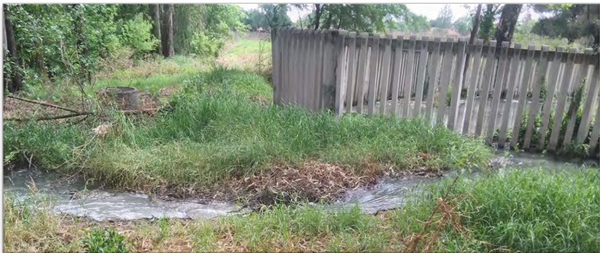
Figure 6.3. Raw sewage flowing into the river, caused by failure of Pumpstation 8 in Vereeniging (taken by Noleen Tavengwa 09/10/2021).
