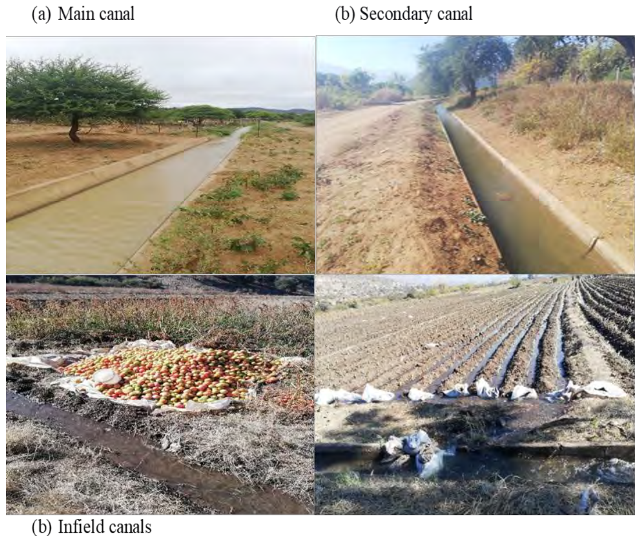
Figure 6.5: Condition of infrastructure in the Tugela Ferry main and secondary canals
