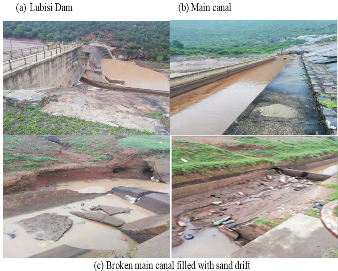
Figure 6.3: Condition of main canal infrastructure in Qamata irrigation scheme
