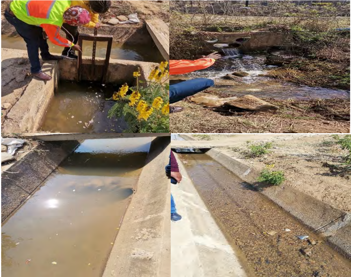
Figure 6.6: Condition of infrastructure in the Mooi River scheme
