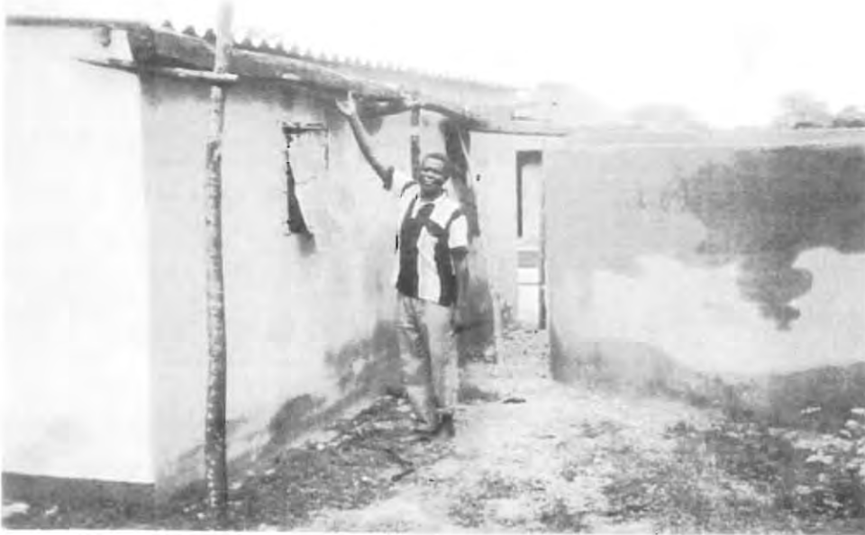
Water harvesting: The rain water harvesting tank at the Ndlovu homestead. Mr. M. Ndlovu shows the guttering which he improvised from local timber.
