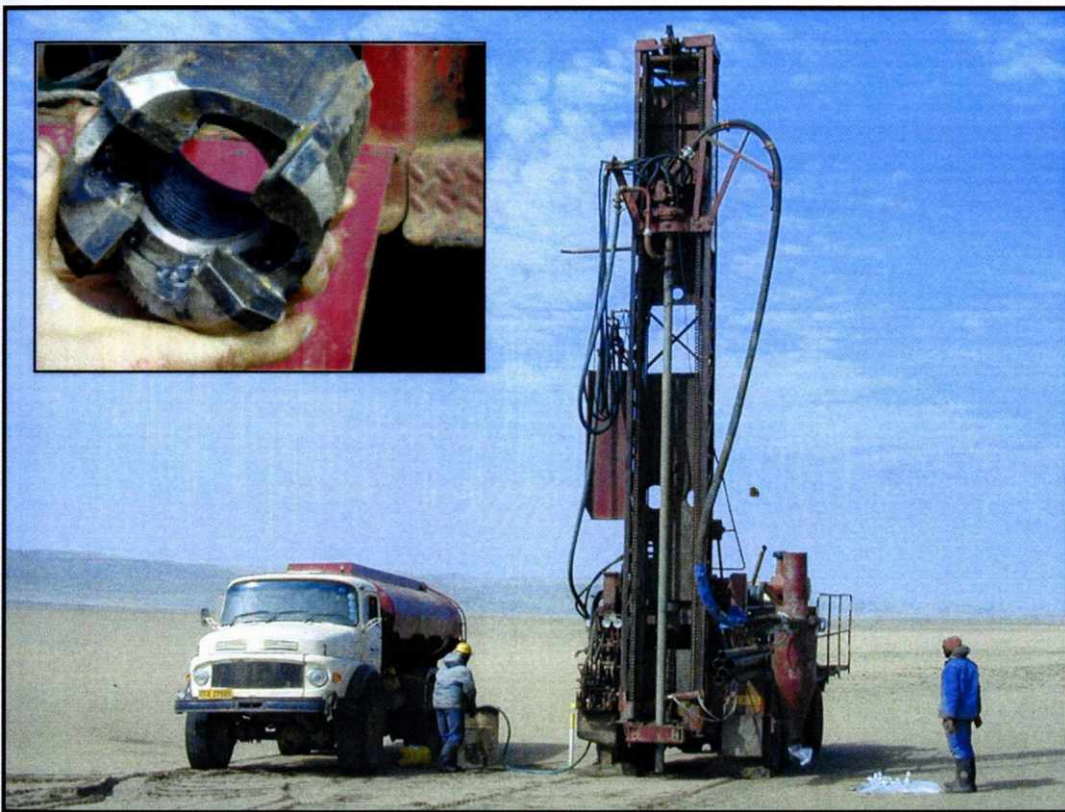
Figure 3.3. The mud drill rig used to conduct small diameter delineation drilling at pocket beach Sites 2 and 3. This drilling constituted the first phase of a recent (1997 to 2002) evaluation programme. The inset shows a hollow-core bit that was used.
