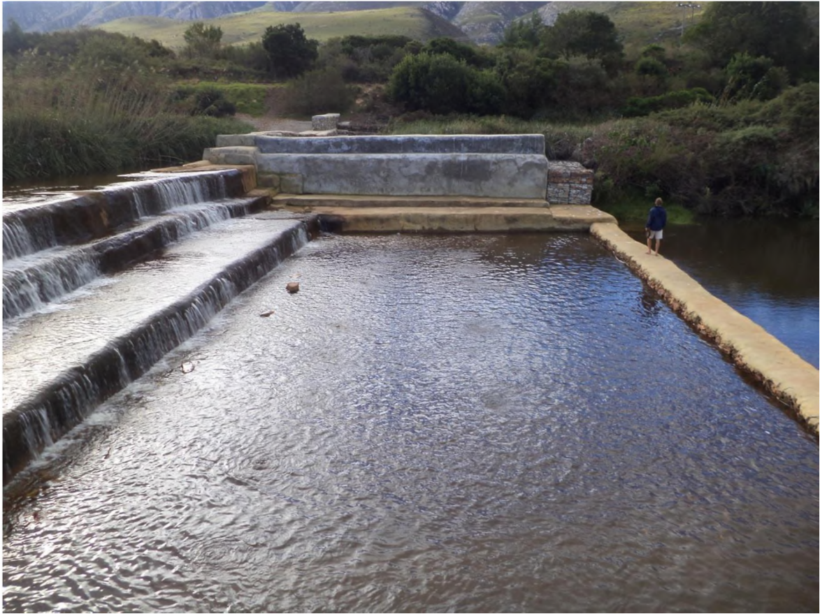
Figure 3.4: A gabion structure installed by Working for Wetlands in the upper Kromrivier wetland, above the Kompanjiesdrif basin, built to restore the river by stopping the headcut from proceeding backwards up the river.
