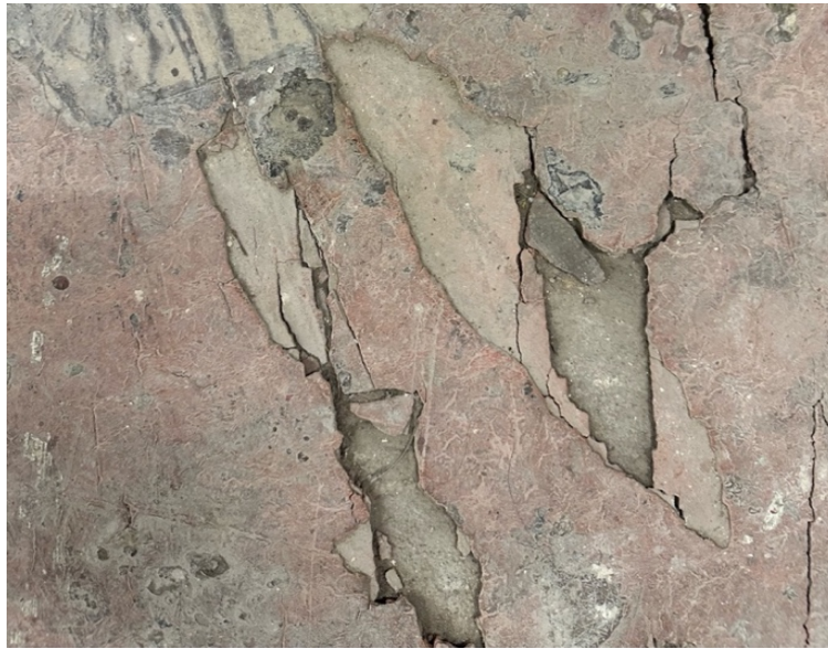
Figure 1: Floor surface cracks and wear serving as source material.
