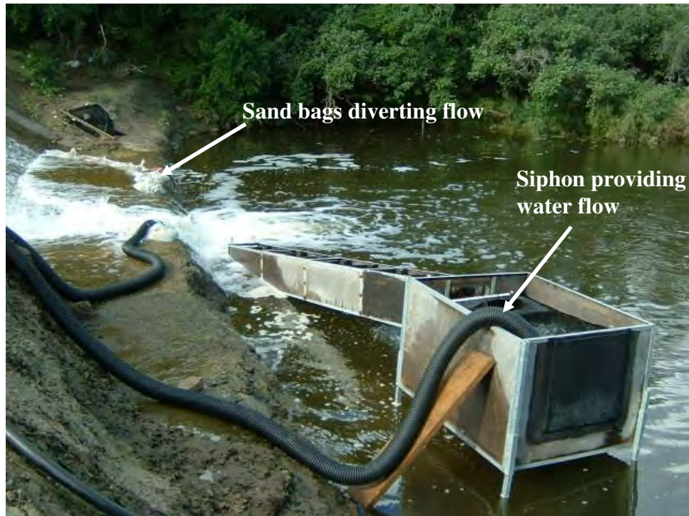
Plate 2.5: Vertical Slot Fishway position 3, below lower apron of weir with water diverted towards entrance with sand bags.
