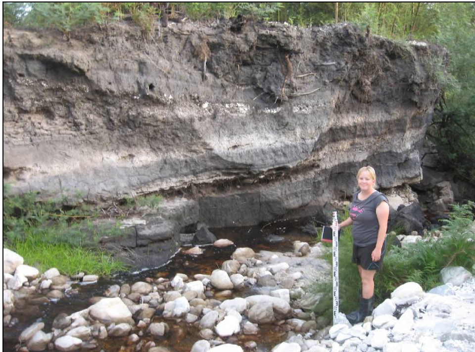
Figure 3-3: Photograph showing the erosion down to bedrock that has occurred in the Tierkloof Wetland.
