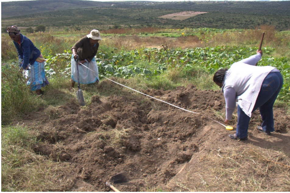
Figure 4.12: Two farmers working with an extension officer measuring the pond and beginning to dig
