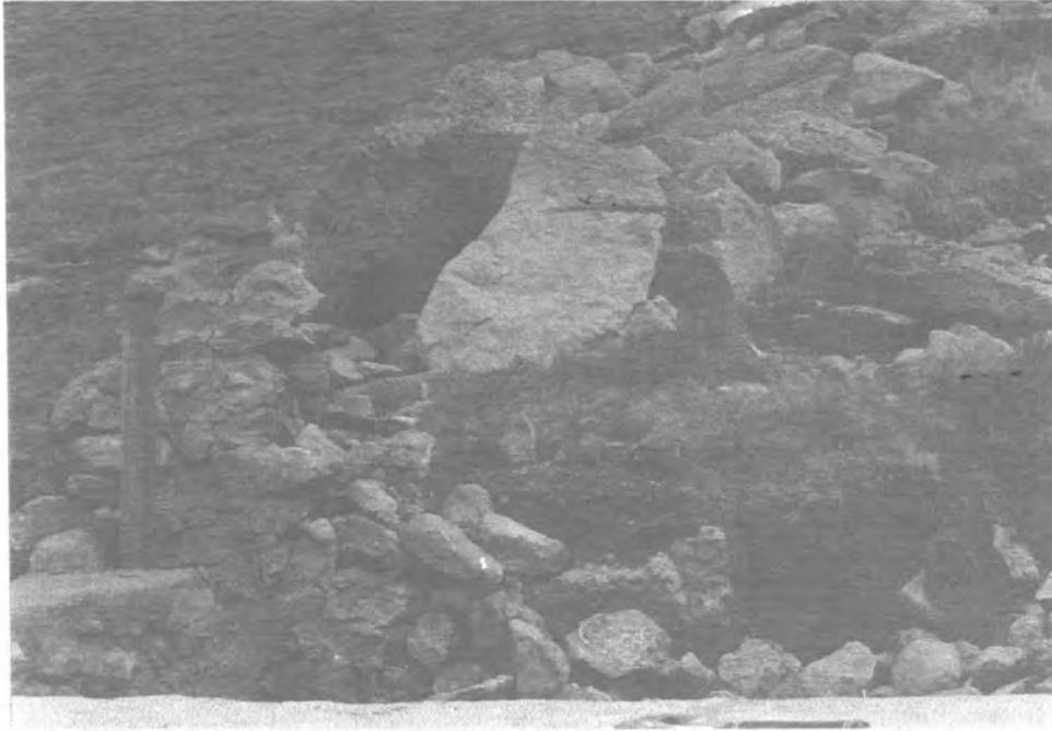
Figure 10.2: Collapse of the upslope wall of the "Ice Pub" (2783m altitude) due to moving gelifluction deposits.
