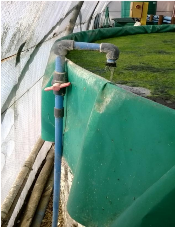
Figure 3.4 The inlet valve used to control the flow of anaerobically digested (AD) brewery effluent into the primary facultative pond (PFP).
