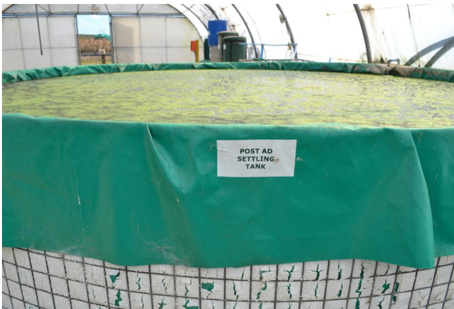
Figure 3.3 The post anaerobic digester settling tank, referred to as the primary facultative pond (PFP) in the text.
