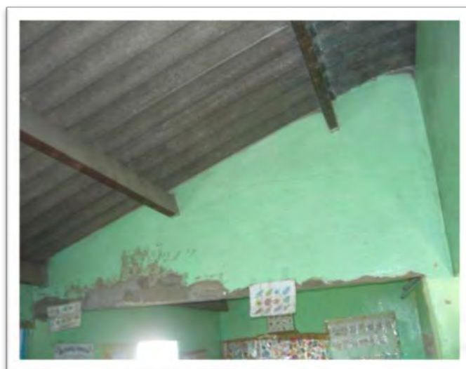
Figure 9: Classroom with no ceiling
