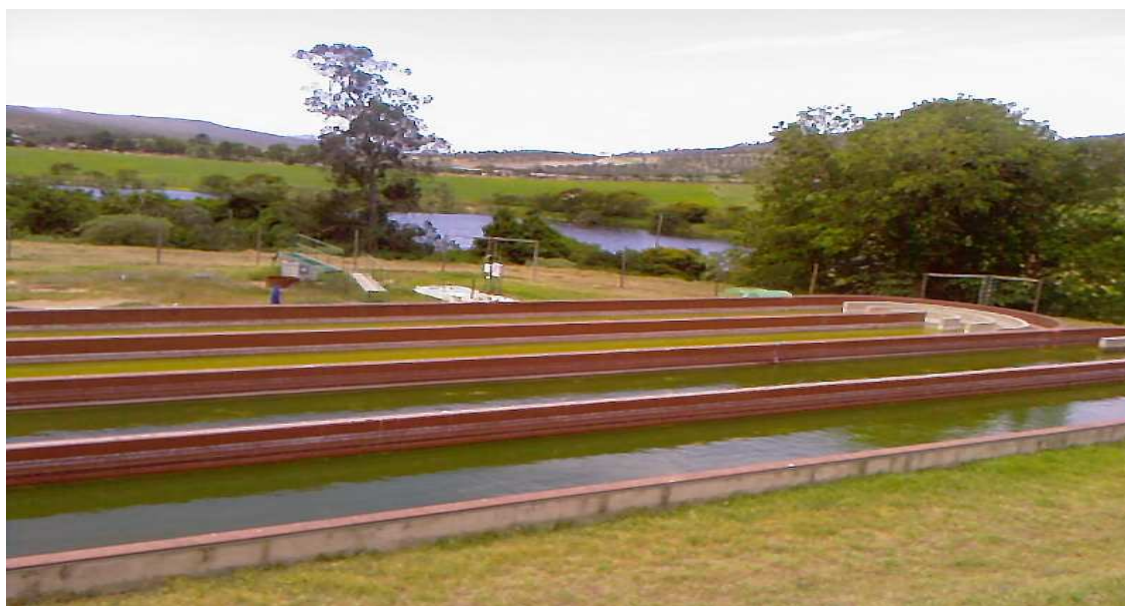
Figure 6.8 Waste Water Treatment plant final effluent before release into a river in the background.
