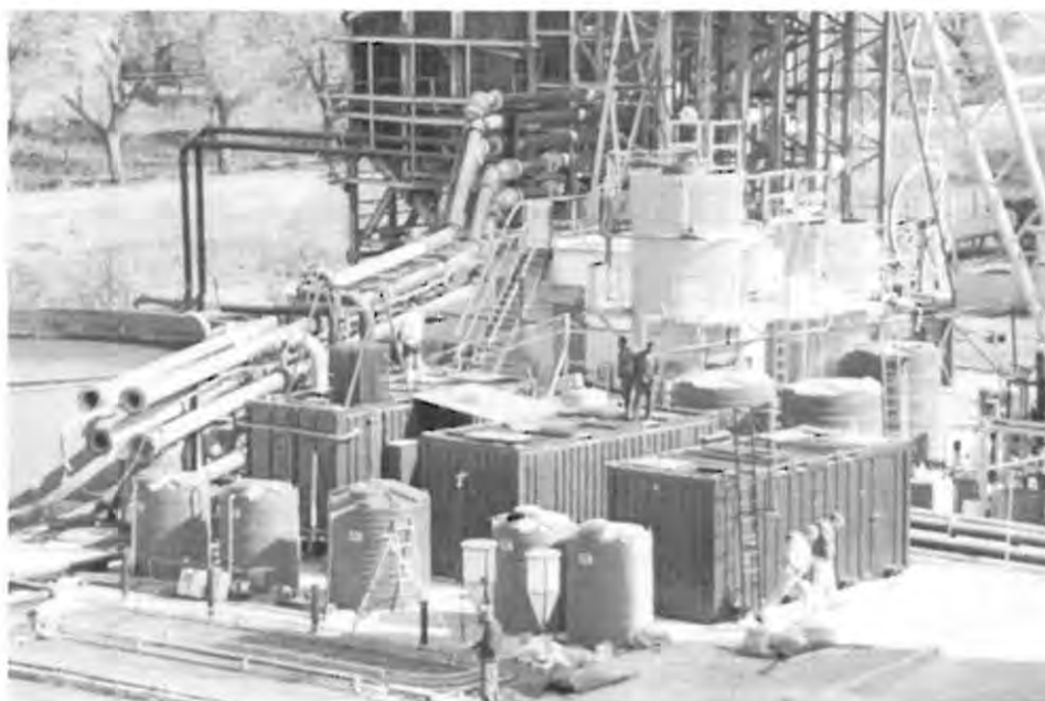
Figure 1.1: The Rhodes 'BioSURE' Process pilot plant at Grootvlei Gold Mine, Gauteng
