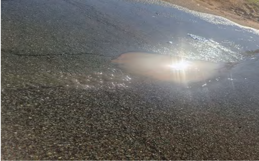
Figure 5.4: A burst pipe causing fissures on the road surface in Refentse
