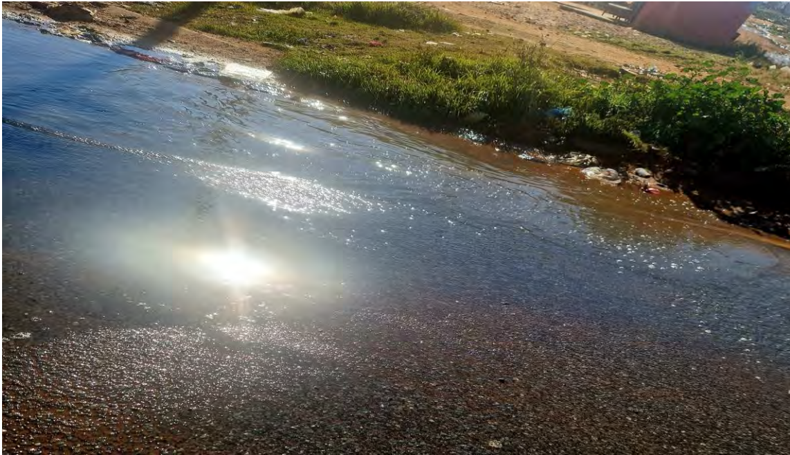
Figure 5.5: A burst sewage pipe in Temba.
