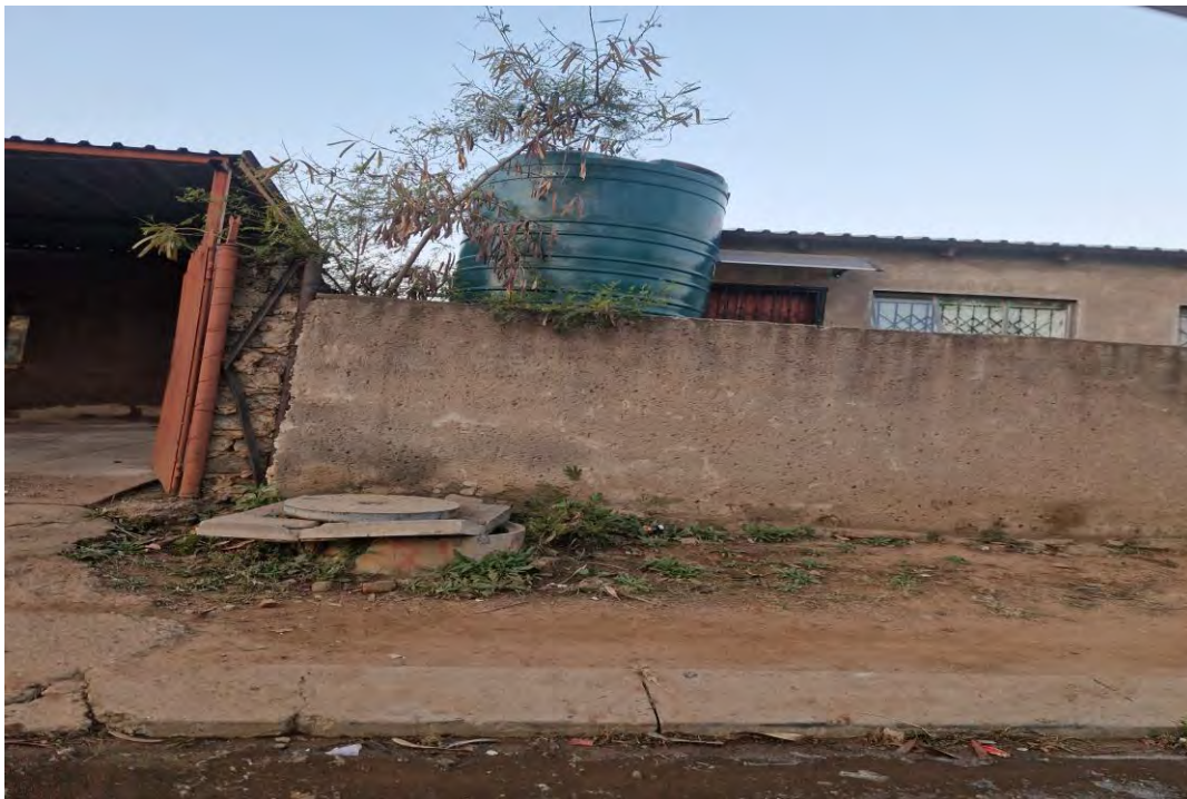
Figure 4.1: House with domestic water storage tank
