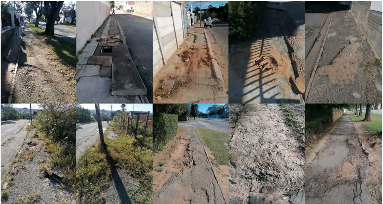
Figure 5.3.7c. An illustration showing poor sidewalk condition within the four study areas.
