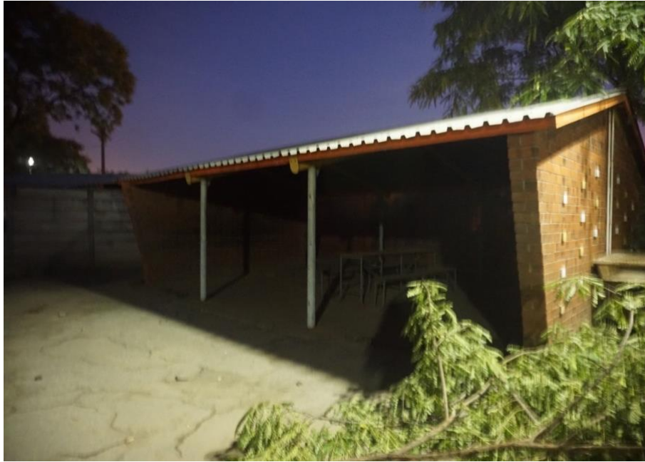
Fig 5.10 Beer garden in decay, former Chiweshe bar, 2018
