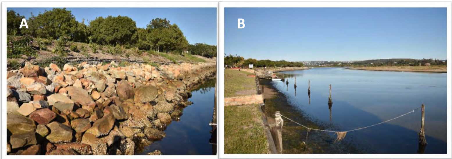
452 Figure 2.1. Artificial erosion control structures found along the eastern channel in the lower reaches 453 of the Keurbooms Estuary. A: rip-rap rocks, B: wooden retaining walls.
