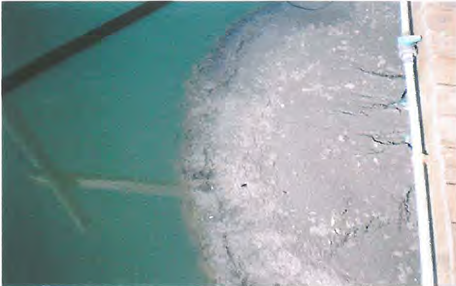
Figure 2.4.6. Active anaerobic sludge visible on top of the gas collector.
