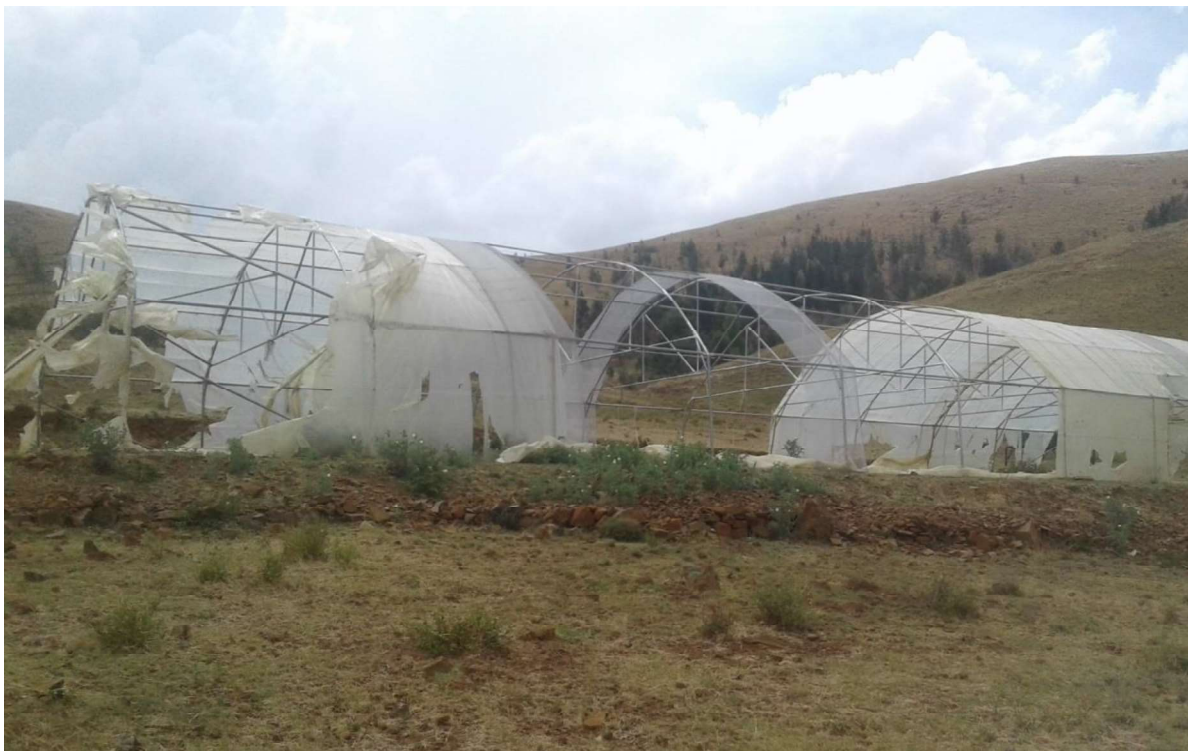
Figure 4.7: Failed greenhouse project funded by the SADP in Ts'akholo, Mafeteng district
