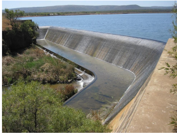
Figure 1.2. The Twyfelspoort Dam wall on the Polkadraai tributary, Groot Marico catchment, North West Province, South Africa.
