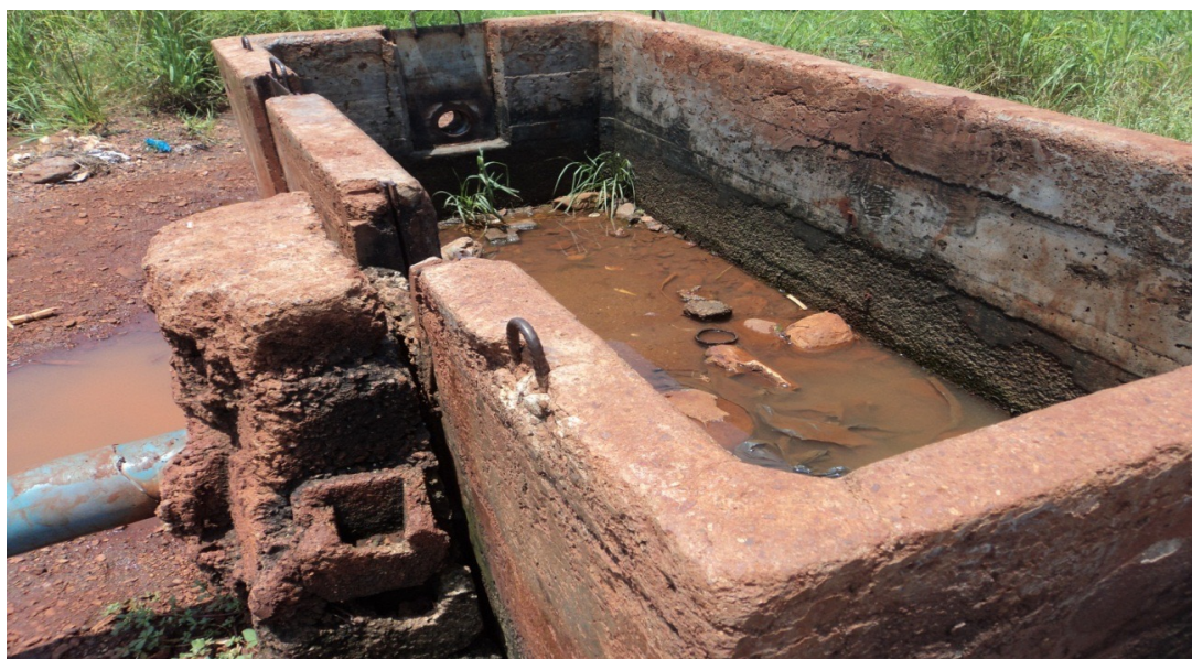
Figure 5.7: Observable disturbances related with poor maintenance and water supply to the field, affecting crop production
