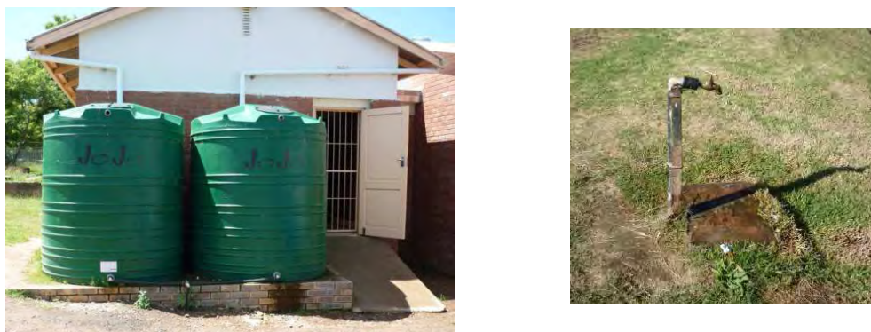
Figure 26: The rainwater tanks and tap at the Eluxolweni Children's Shelter.
