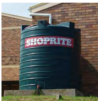
Figure 29: The rainwater tank at Samuel Ntsiko Primary School.
