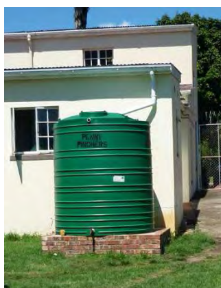
Figure 28: The rainwater tank at the Rhodes University Grounds and Gardens building.
