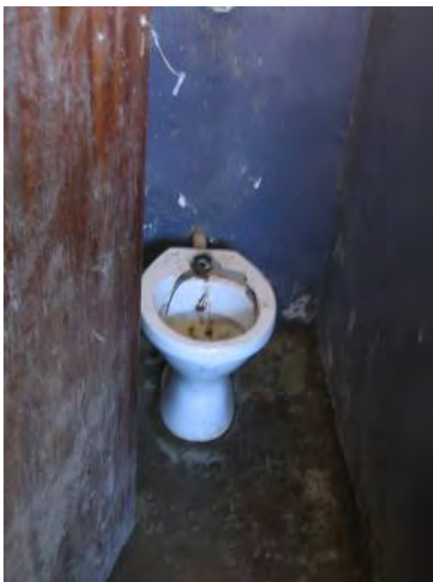
Photograph 79: Broken and blocked toilets
