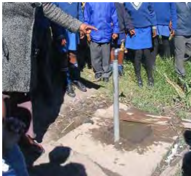
Photograph 81: Teacher points out blocked drain during audit of water waste hot spots
