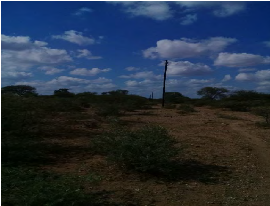
Figure 5. Power lines in rural Mphoengs to service the stamping mills dotted in the district .
