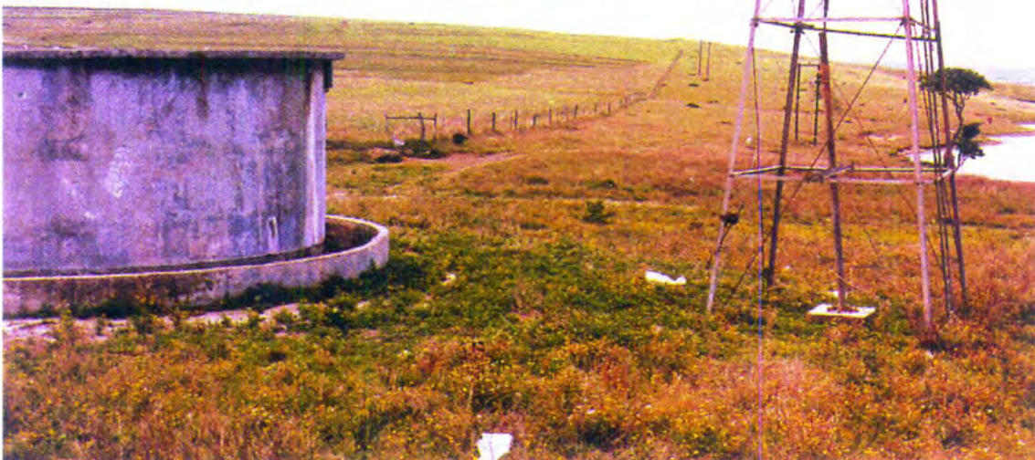
Plate 5: A borehole which had to be abandoned due to nitrate pollution from cattle excrement (the cattle drinking trough is situated too close to the borehole and the borehole itself is inadequately sealed at surface by the too small concrete block).
