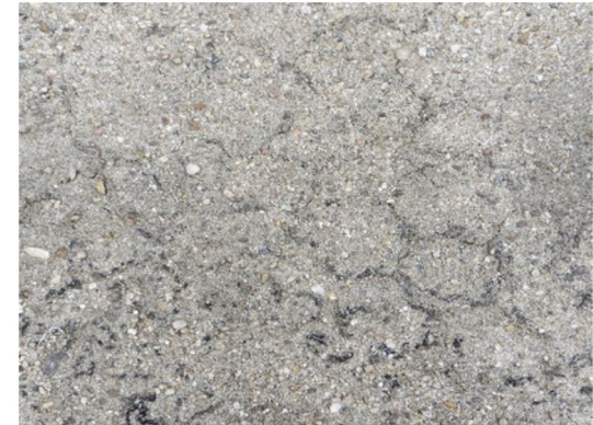
Figure 53: Desiccation cracks (Grjotøya, Antarctica).
