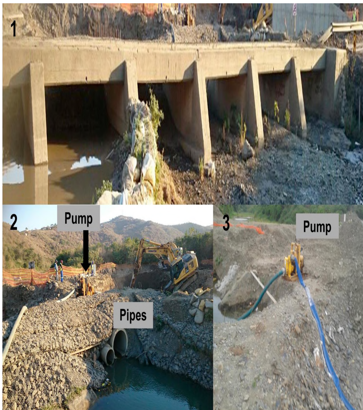
Figure B1: Infrastructure upgrading of the road bridge upstream of the Mngazana Estuary. 1: Old Bridge; 2: Two pipes being used to allow river water to flow into the estuary; 3: During construction, freshwater is also being pumped from the river section into the estuary via the pump. (Images: Cotiyane 2015).
