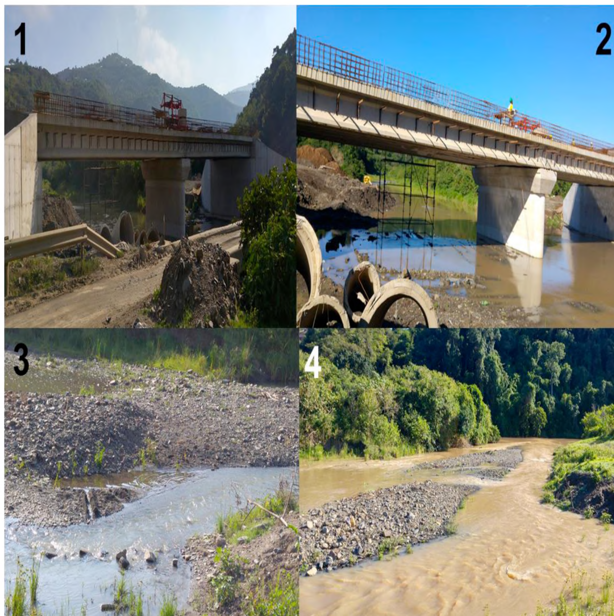
Figure B3: Construction progress on the infrastructure upgrading of the road bridge upstream of the Mngazana Estuary (March 2016). 1 & 2: New Bridge is near completion; 3: Freshwater inflow increased marginally from June 2015 to March 2016; 4: and substantially after a rainfall event which may affect the turbidity of the estuary (Images: Dr Rajkaran 2016).
