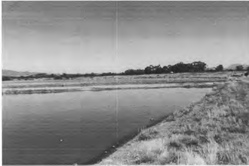
Figure 2.4.7. Photograph of the 'red' anaerobic ponds in the waste stabilisation ponds at Mossop Western Leathers, Wellington.
