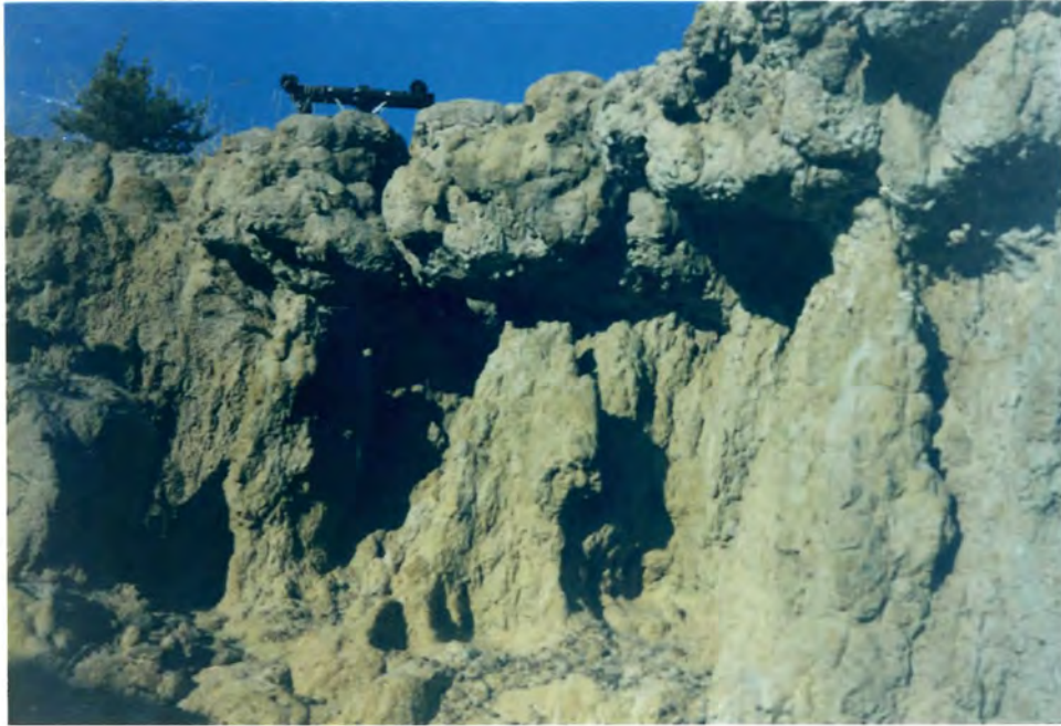
Plate 9 Gully wall showing undercutting of the subsoil.
