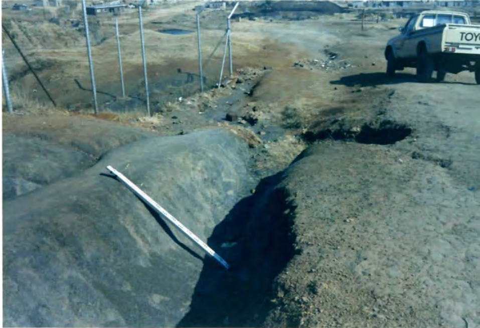
Plate 7 Road drain developing into a gully.
