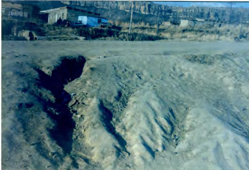
Plate 5 Extensive rilling on road surface.
