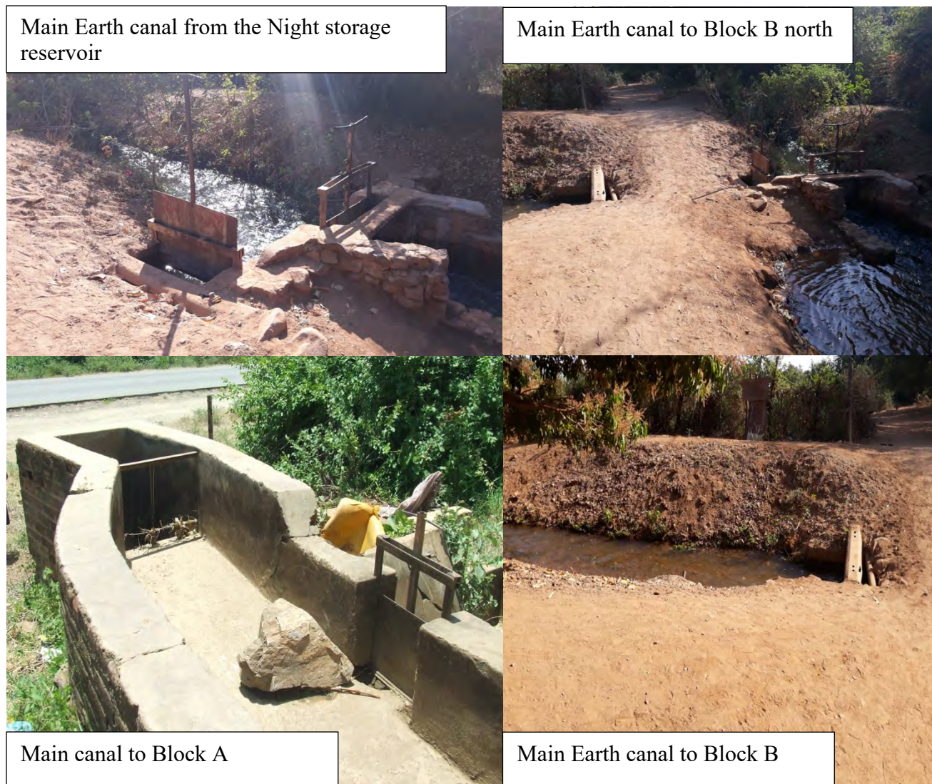
Figure 3.1: Earth silted canals and leaking, broken canals.
