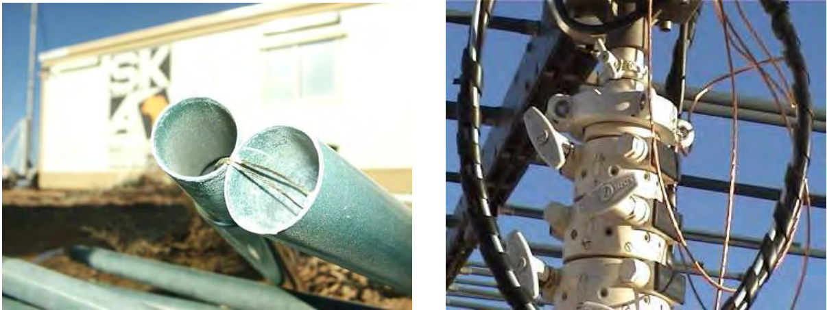
Figure 4.3: Left: The metal chain inside the gazebo poles which caused interference at the Karoo 3 core site. Right: Initial earthing of the mast segments using copper wire. Note the guide-rope collar which is still attached to the mast at this stage.
