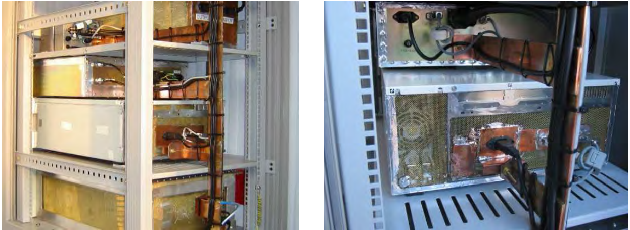
Figure 4.4: Left: The trailer rack with the measurement system equipment installed and the cables strapped to the copper busbar. Right: A close-up view of the busbar attached to the Electronics Control Box and Control PC.
