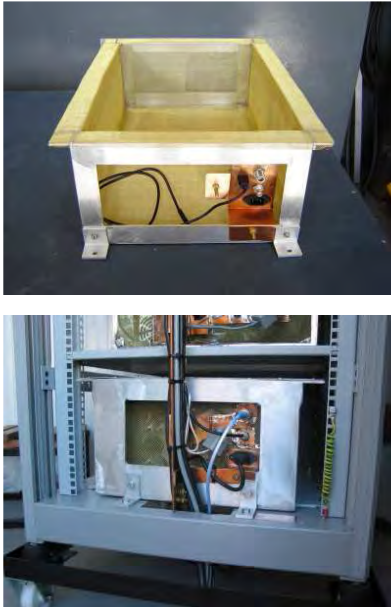
Figure C.2: Top: Spectrum analyser Faraday cage with bulk-head connectors, mains filter and copper flange for attachment to the copper busbar. Bottom: Spectrum analyser installed in the trailer rack with power and control cables strapped to the busbar.
