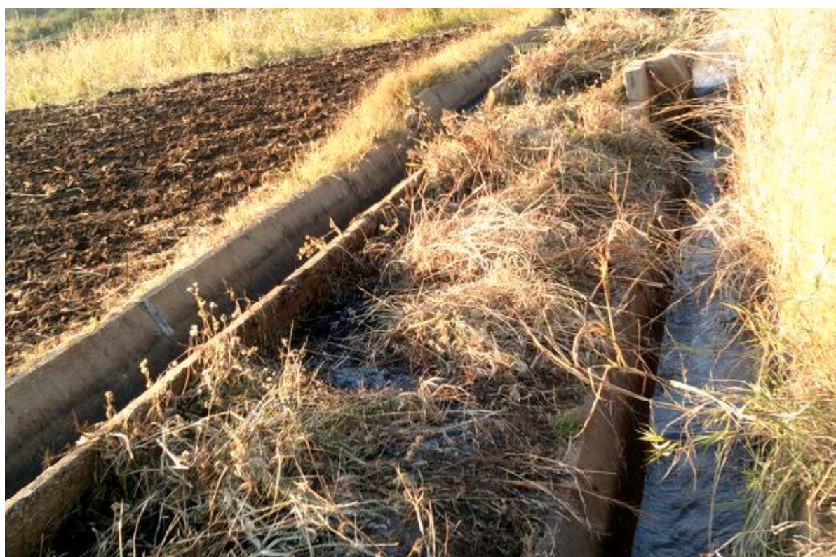
Figure 12: Secondary and Tertiary Canals Requiring Cleaning Up and Repairs
